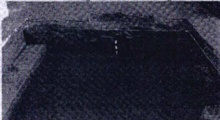
Reused brick structure just below the random uneven sized boulders - During - closer view - Section facing north
